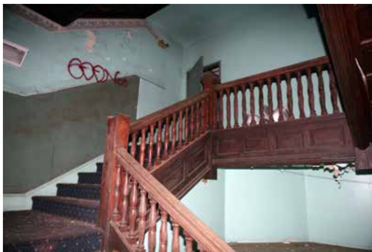
Photo: Courtesy of Heritage Investment Corporation This photo of the interior stair of the Nugent Home for Baptists shows the results of a decade of abandonment and decay.
